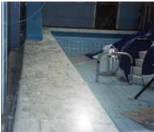
Figure 1.7 Uncontrolled removal of asbestos
