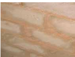
Figure 7.26 Remnants of asbestos on breeze blocks
