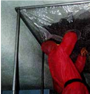
Figure 7.17 A sprayed asbestos coating being removed using a specialised glovebag within a traditional enclosure (the dark area is where the asbestos has been removed)
