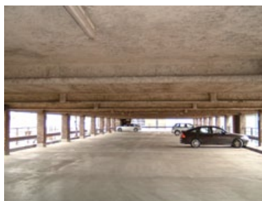
Figure 7 Sprayed limpet on car park roof
