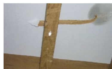
Figure 25 Chrysotile paper on strawboard ceiling panels
