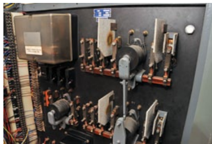
Figure 50 Open electrical switchboard with asbestos flash guards
