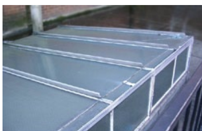
Figure 31 Chrysotile string on skylights
