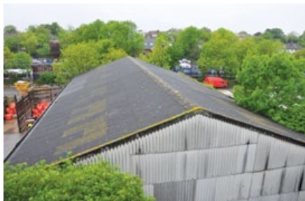
Figure 32 Asbestos cement roof and wall cladding
