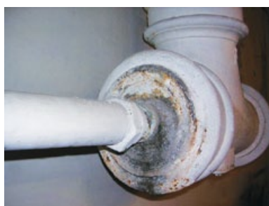
Figure 30 Amosite and chrysotile packing on waste pipes
