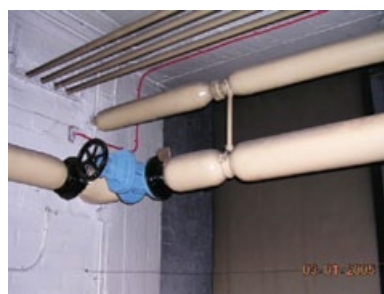
Figure 4 Pipe uncertainty: Top pipe is non-asbestos. All pipes should be sampled
