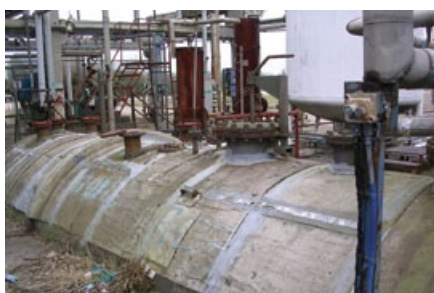
Figure 12 Lagging on large petrochemical vessel
