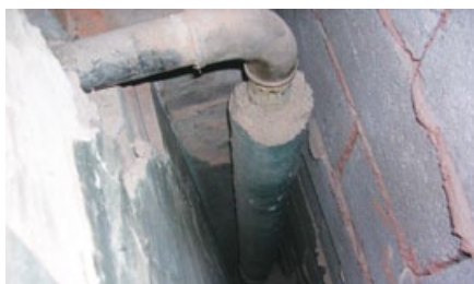
Figure 9 Lagged pipe in wall cavity
