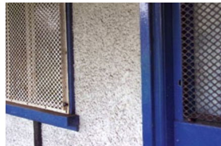
Figure 33 Chrysotile pebble-dash exterior wall coating
