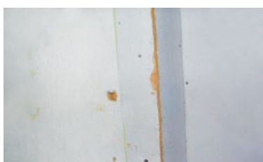
Figure 24 Chrysotile paper on fibreboard boxing
