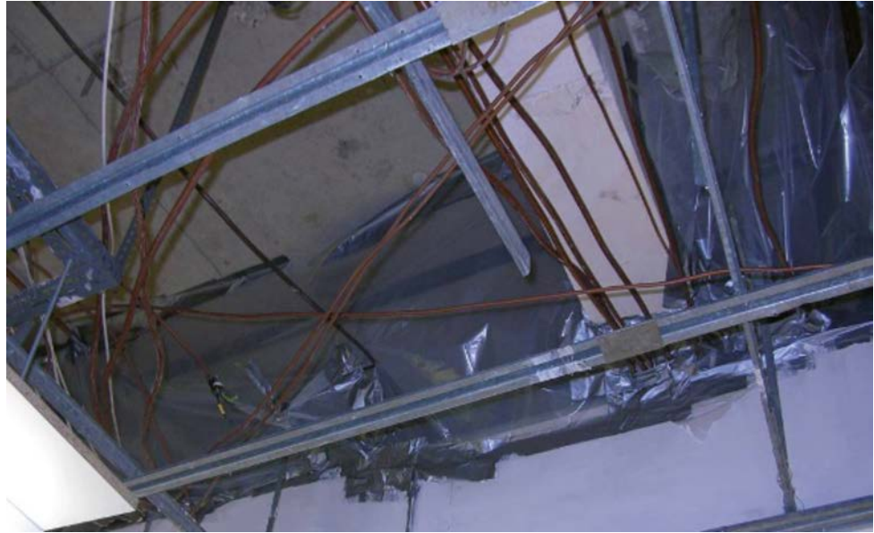
Figure A5.4 Void photo showing locations and extent of surfaces, cables and other items that need to be visually inspected for dust and debris
