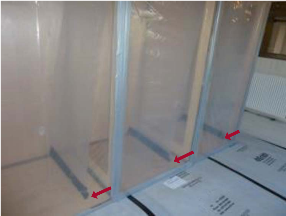
Figure 5.7 Airlock door flap deflection of 200–250 mm in chambers 2 and 3 at the base of the flap (see arrows) indicates that the NPU is extracting 1000m 3 /hr and enclosure internal negative pressure is –5 Pascals (see Asbestos enclosure ventilation research ) 38
