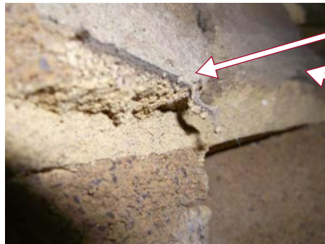
Figure A5.9 Remnants of asbestos on materials
