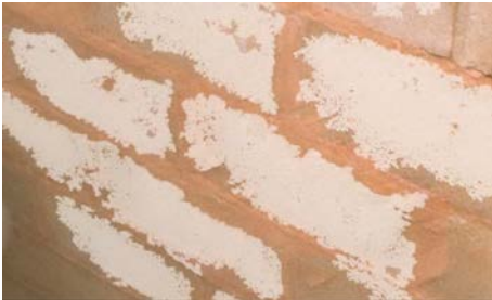
Figure A5.10 Remnants of asbestos on breeze blocks
